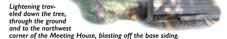
Lightening traveled down the tree, through the ground and to the northwest corner of the Meeting House, blasting off the base siding.
