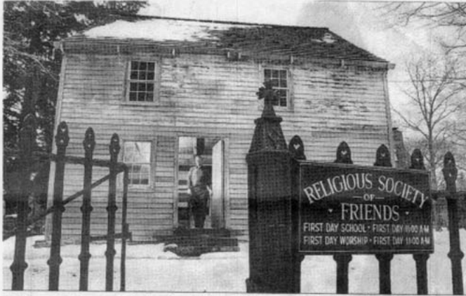
Hal Haydock stands in the doorway of the meeting house. Exterior paint stripping completed and ready for linseed oil finish in spring of 2004.
